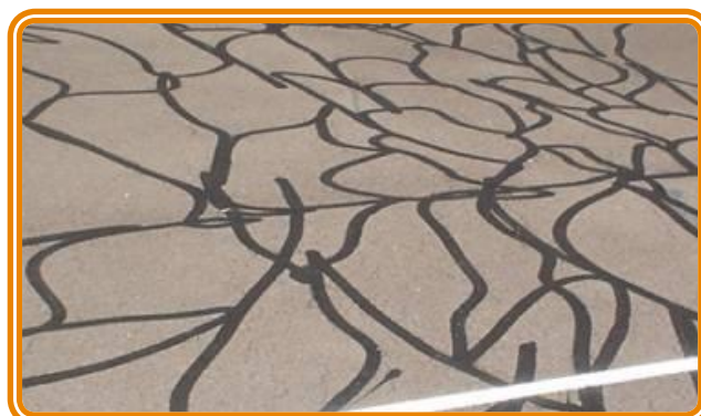
Cracked court filled with Liquid Bitumen Emulsion
