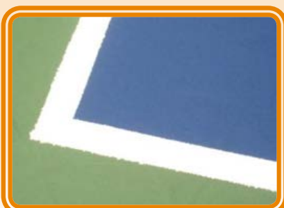
Line marking allowed to ‘Bleed’ under the tape
